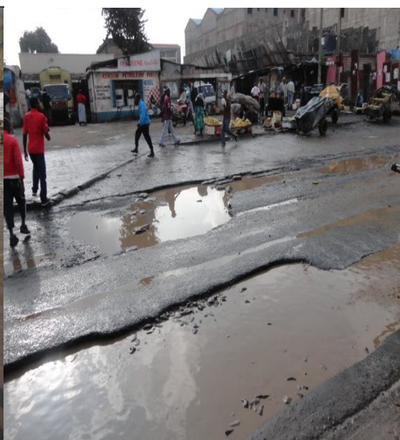
Plate 2: Dilapidated status of main Roads Source: Field Surevy, 2012
