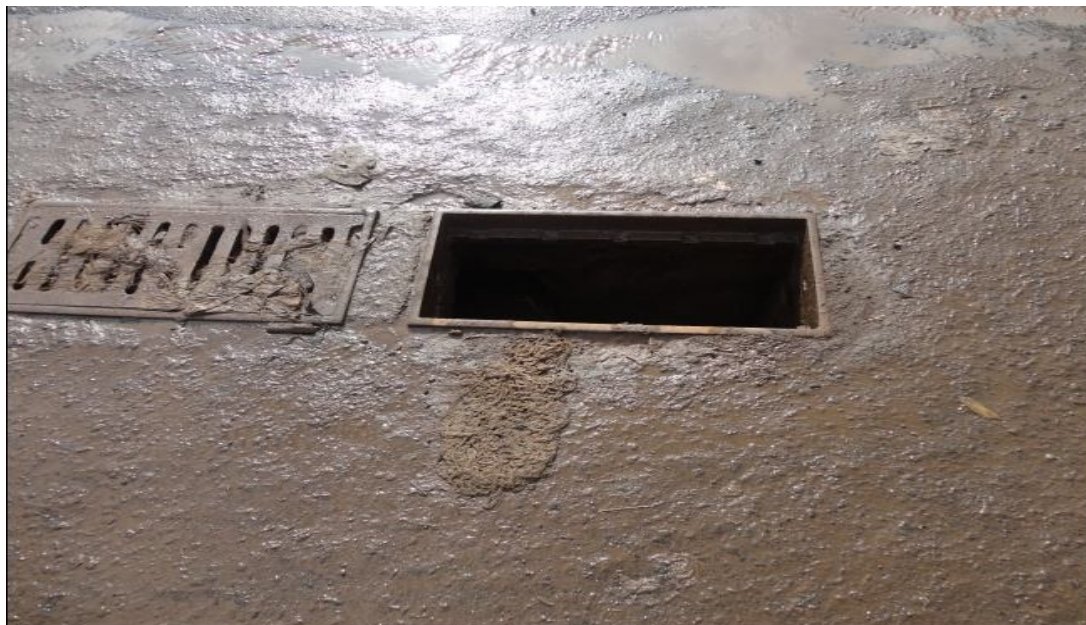
Plate 3: Vandalized storm Water drainage manhole cover
